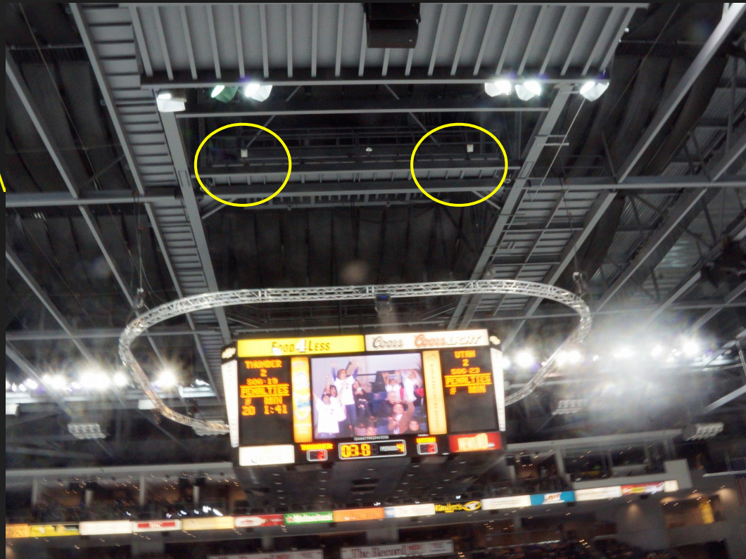
APs mounted on catwalk about 55 feet above the ice.
